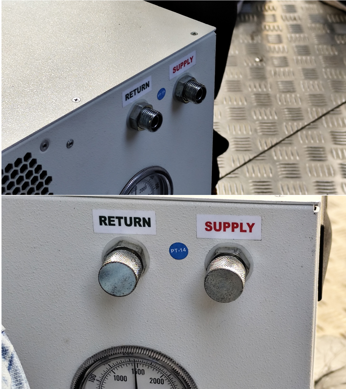
Figure 5: Top to bottom: The compressor supply and return ports after removing the cables. Same ports after putting on the caps.
