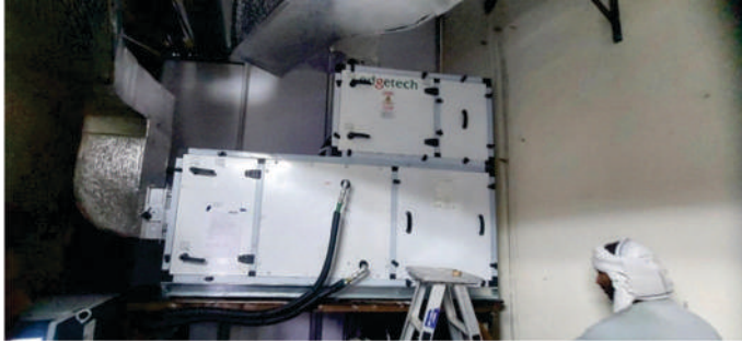
Figure 82. Smart AHU (1200cfm with PID flow modulation).
